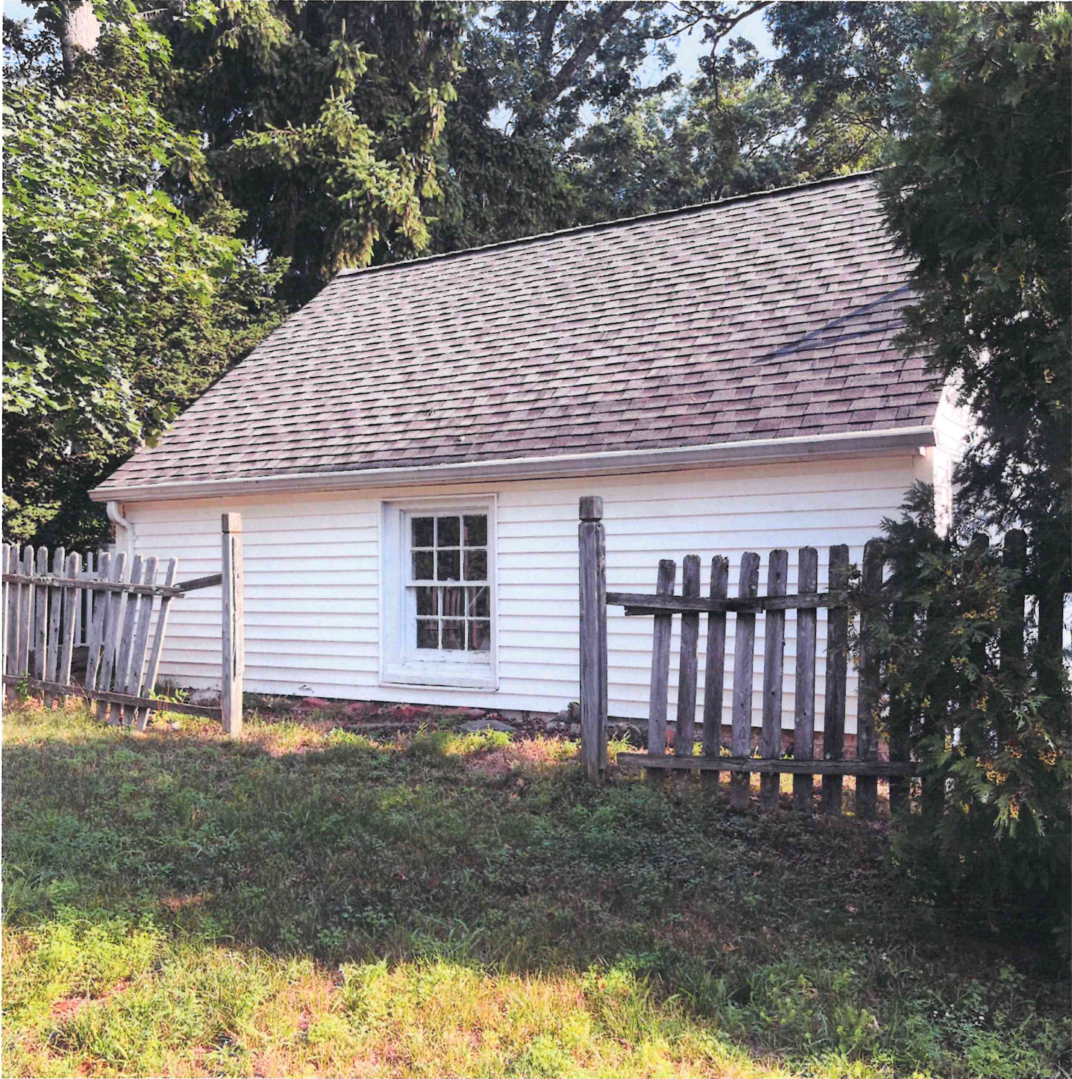
Photo C 8/1/24 photo of neighbor's garage on Lot 9 to north. Fence to be removed and arborvitae planted.
