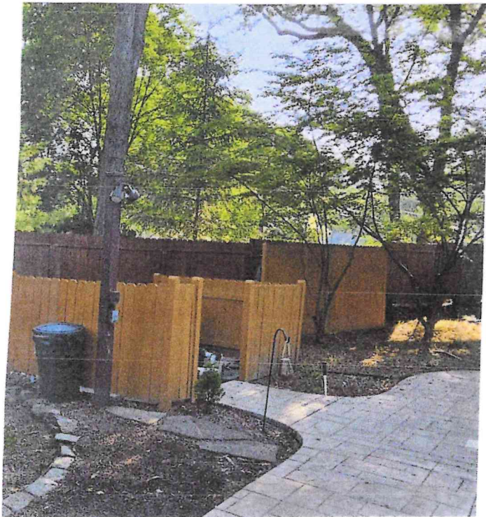
FIG 7 FENCE AROUND POOL MOTOR
